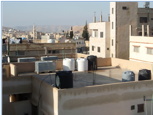
Water tanks on rooftop in Zarqa
