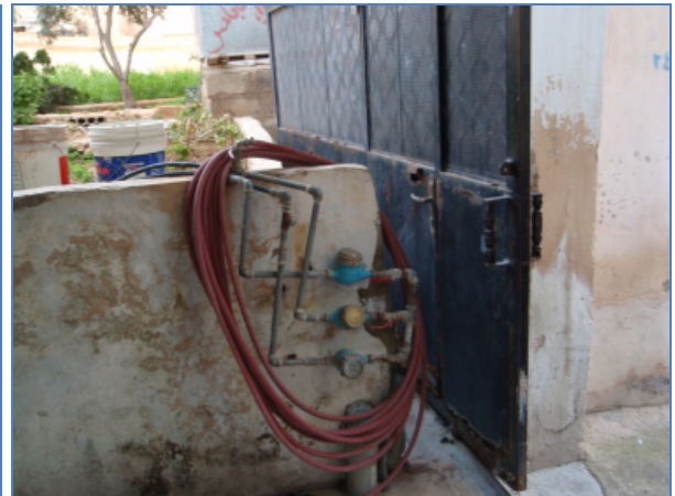
Separate water meters on house with three individual flats in Zarqa
